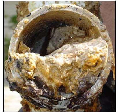
Sewer line inundated with grease
