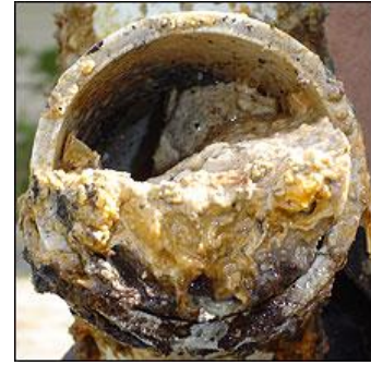
Sewer line inundated with grease
